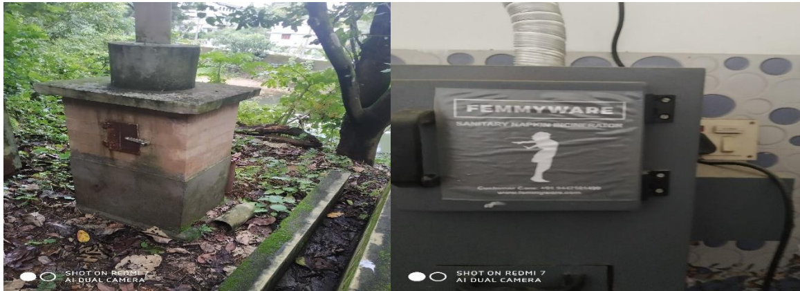
Figure 2: Incinerator in college and ladies toilets
