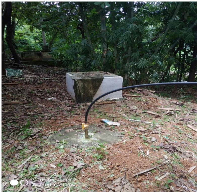
FIGURE 1: BIO GAS PLANT
